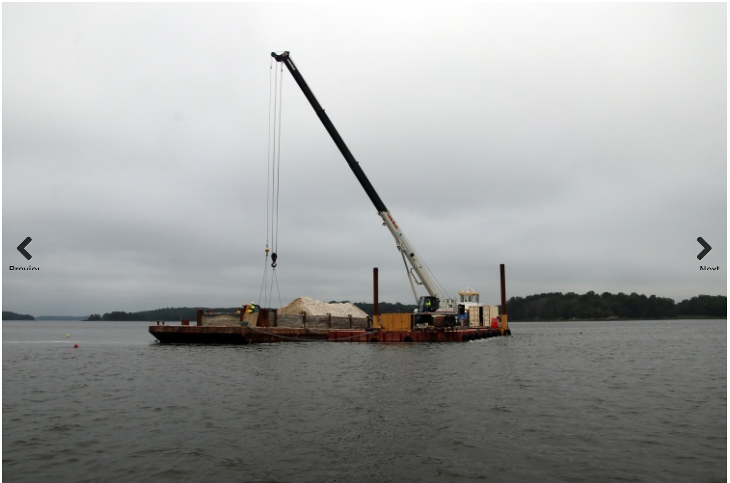
A barge and crane operated by Riverside & Pickering Marine Contractors deposits seasoned oyster shell at an oyster restoration site near Nannie Island.
