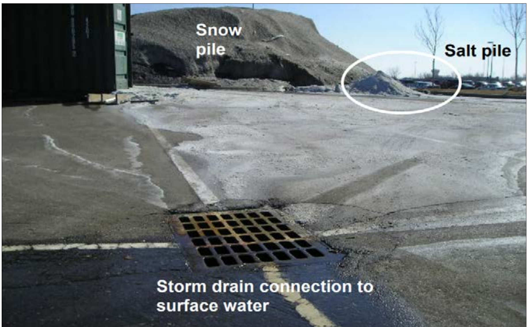
Photo courtesy of UNH's The Winter Parking and Sidewalk Maintenance Manual: Demonstration of Incorrect Salt Storage.
