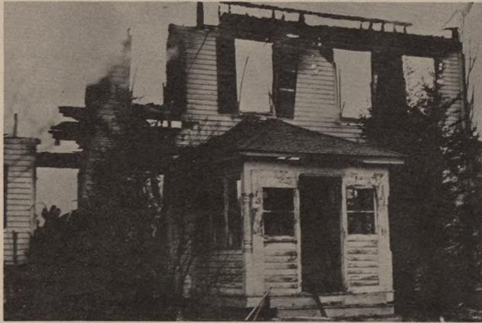
The frame of the apartment house on Mast Road after fire pitted it Monday.
