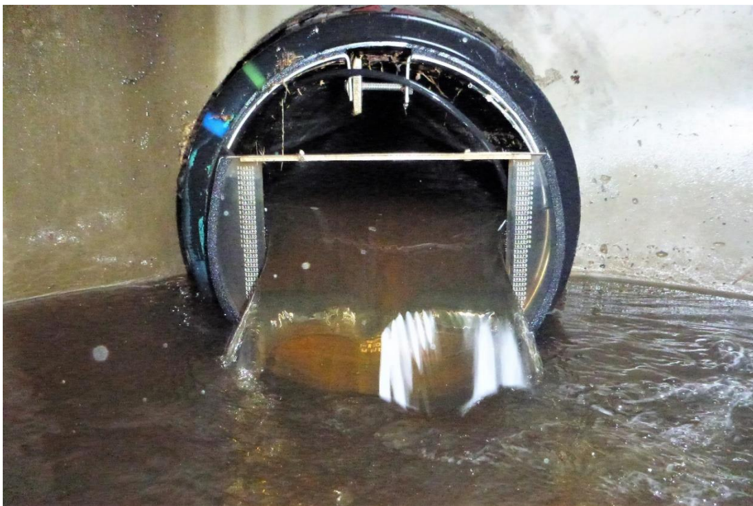
Figure 15: Outlet monitoring using a 12 inch, Thel-mar volumetric weir
