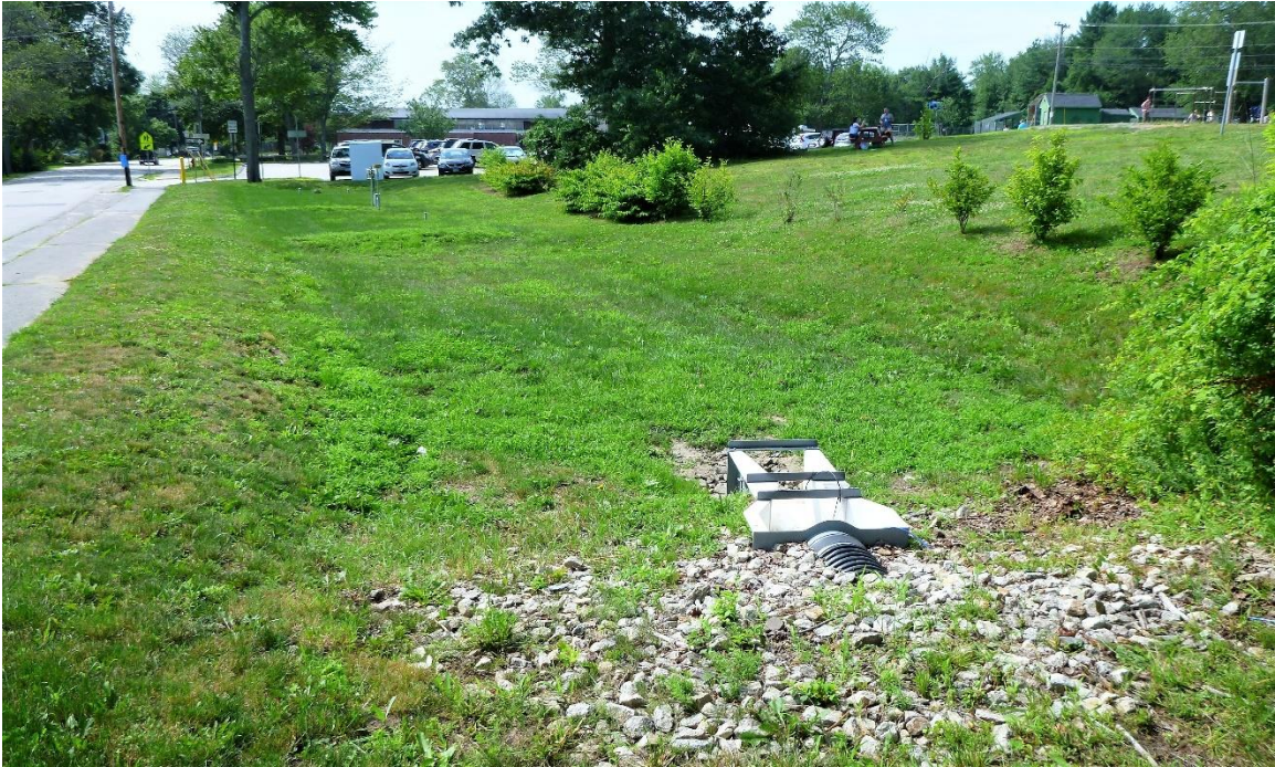
Figure 12: Horne St. bioretention system with viewed from the North, showing the inlet.
