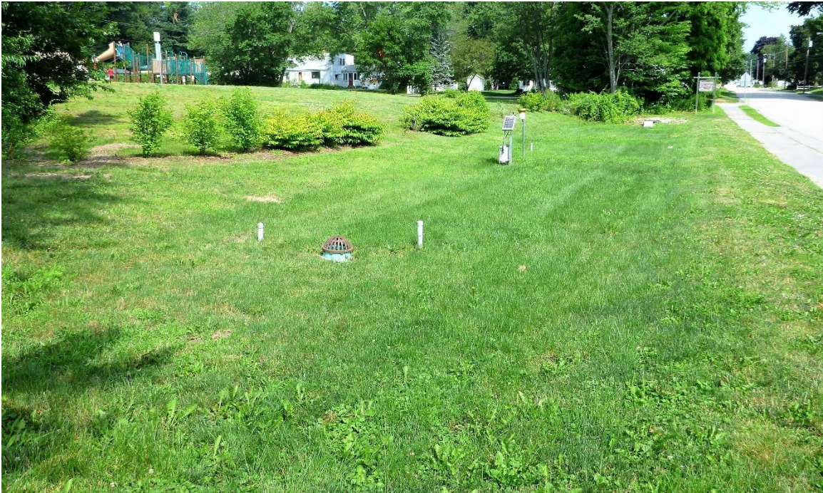
Figure 13: Horne St. bioretention system viewed from the South showing the high-flow bypass and two wells with P41 and P42 pressure transducers.
