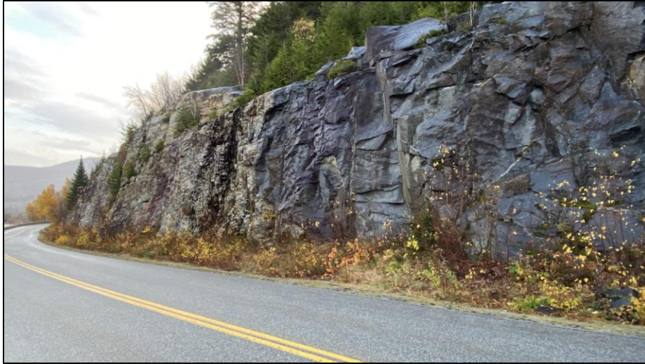
Figure 5.14. Road cut with low safety conditions to conduct rockfall tests in Franconia NH.
