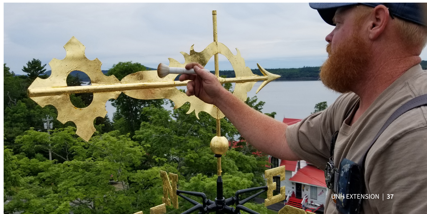
Mid-Maine Restoration finishing the weathervane on the Sewall Memorial Congregational Church, Robbinston, ME. Photo: Maine Preservation.
