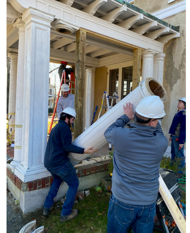
Porch restoration at the First Amendment Museum, Augusta, ME. Photo: Maine Preservation.
