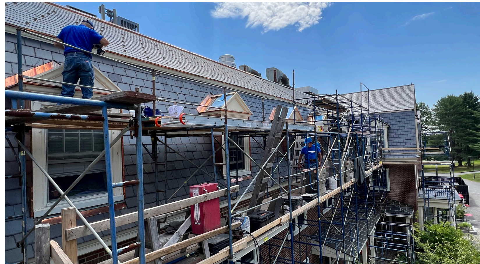
Slate roof restoration by The Heritage Company, Colby College, Waterville, ME. Photo: Maine Preservation
