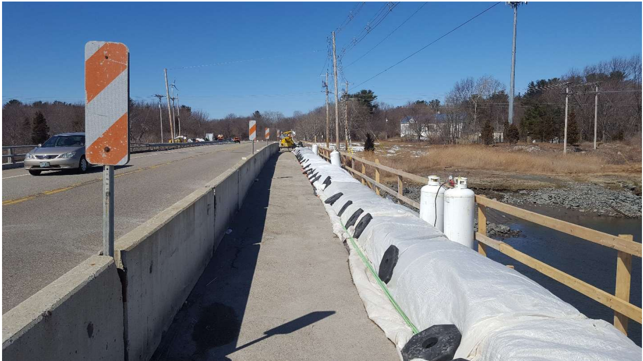
Figure 7: Insulated wrap and heaters on a bridge curb after cold weather placement.
