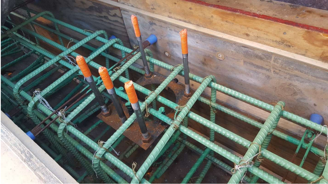
Figure 6: Guardrail anchorage and reinforcement in curb formwork. Tape on the top of the anchoring system keeps threads clean during concrete placement.
