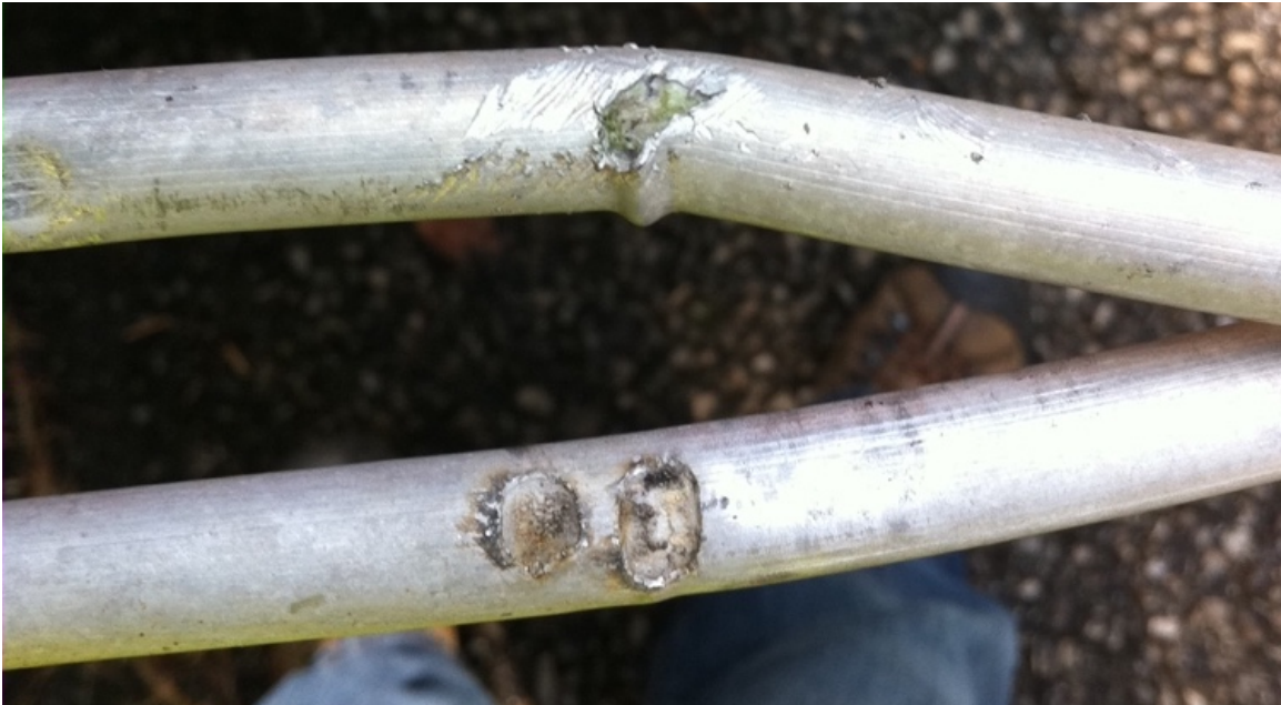
Fig. 2. Abrasion from wind motion (top) and holes from electrical arcing (bottom)
