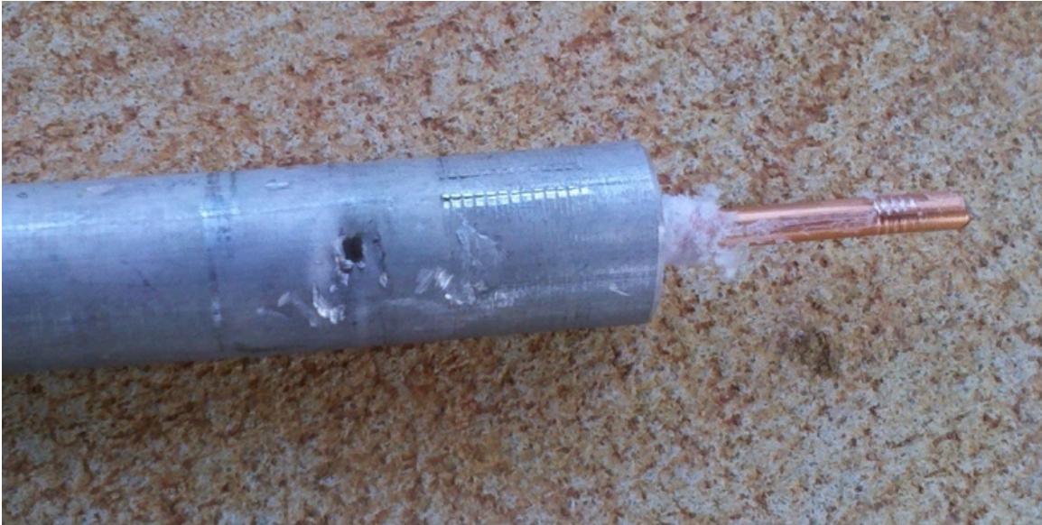
Fig. 1. Small (~2mm) hole in 0.500" coaxial cable caused by tooling
