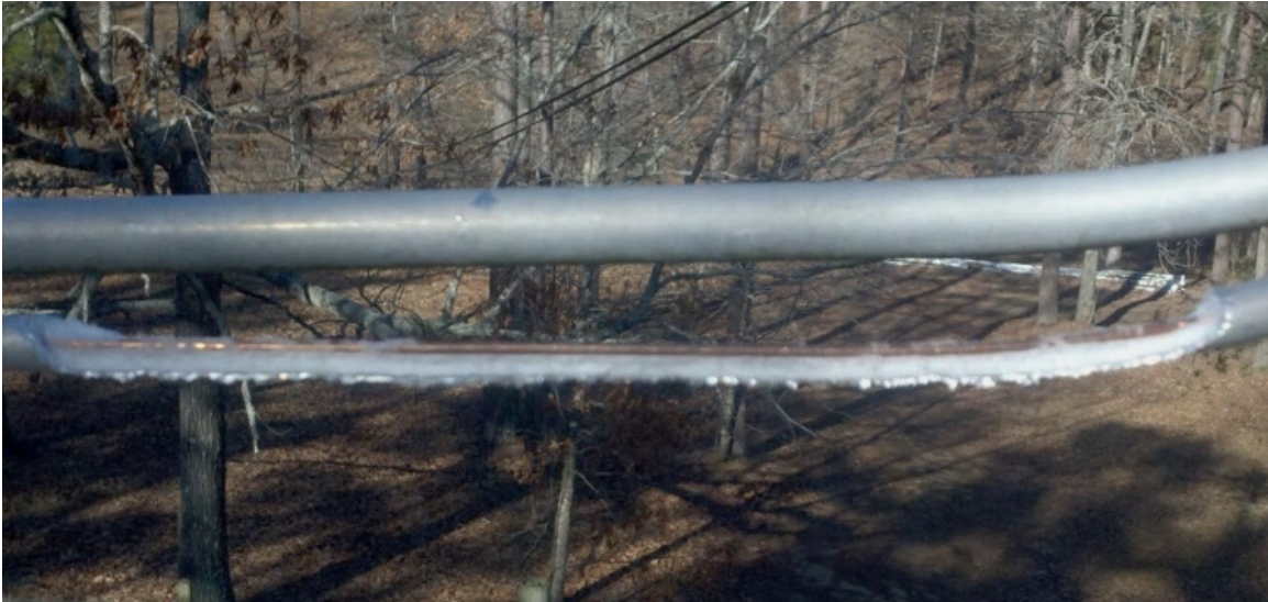
Fig. 10. Squirrel-damaged coaxial cable in an HFC network
