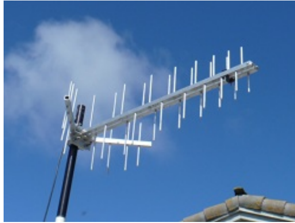
Figure 3.5: The new Stoke Hall sector antenna
