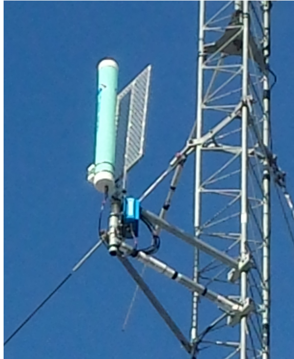
Figure 3.4: Kingsbury Hall omnidirectional antenna with reflector
