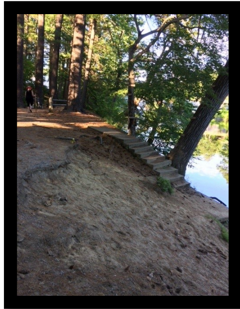
Work to be Done: Immediate attention is needed to repair the erosion of the riverbank near the rope swing.
