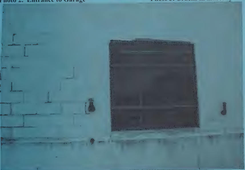
Photo 4: Window deterioration and cracks in block masonry and foundation
