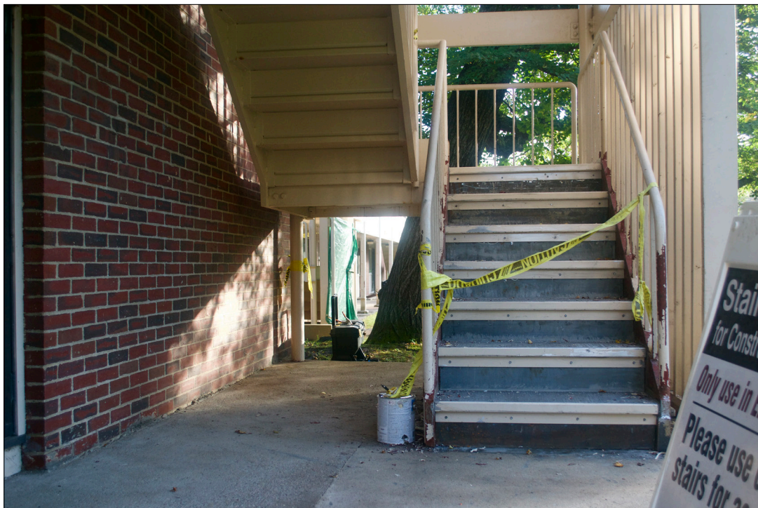
A Forest Park staircase under repair so the apartments can remain suitable for living until demolition.
