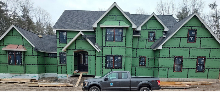
A new residential build. The Building Inspectors will conduct over a dozen inspections, from start to finish.
