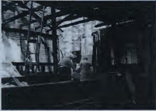
Two citizens inspect the remains of the meetinghouse. Intact end wall, ceiling joists and one tie beam visible. Box and bench pews survived.
