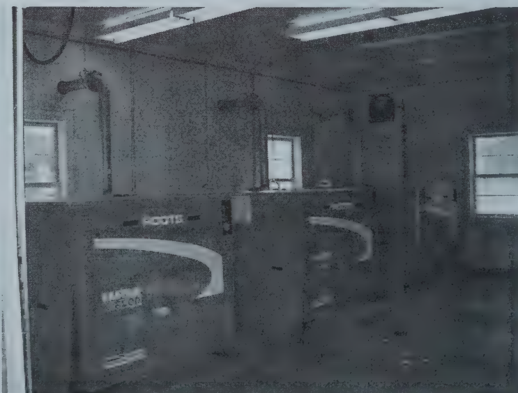
The new aeration blowers. Photos courtesy of Ken Levesque.
