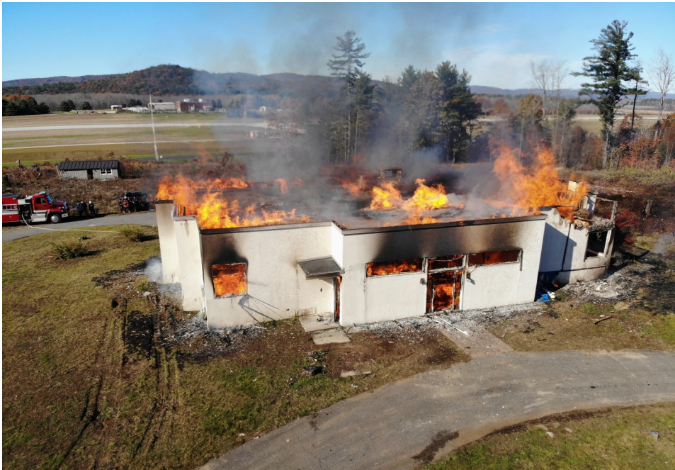
Controlled burn for training and demolition of the building at 321 Old Homestead Highway on Saturday November 6th.
