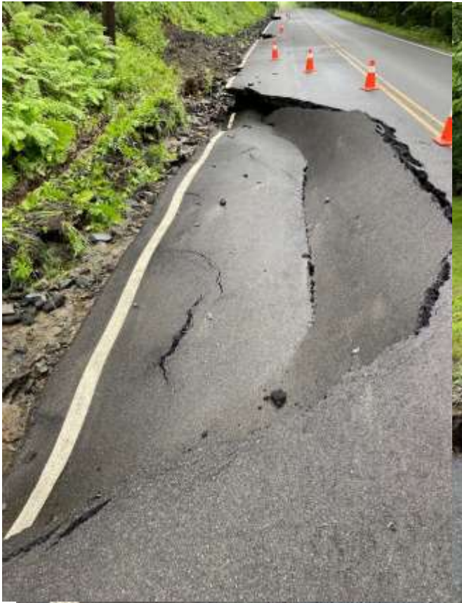
Stevens Road Storm Damage, July 2023
