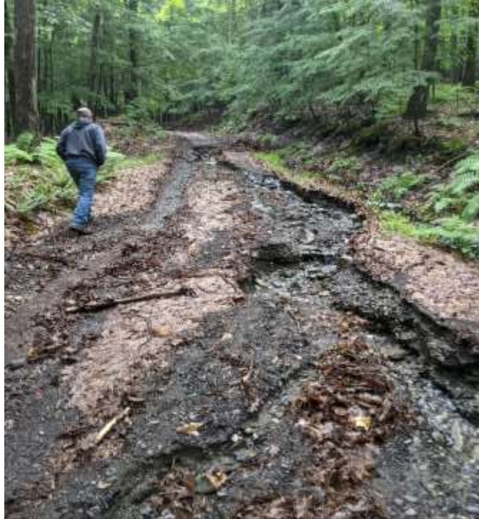
Washout on Balch Hill Tank Access Road
