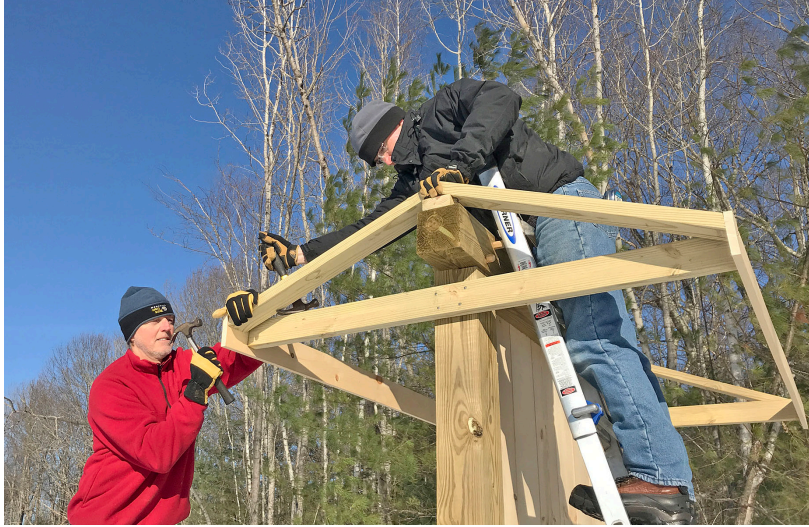
Conservation Commission members John Nachilly and Rob Sullivan work on the kiosk roof at the Thompson Forest where trail maps and information about the properties will be posted. The kiosk was funded by the Lamprey River Advisory Committee. Courtesy Ellen Snyder
