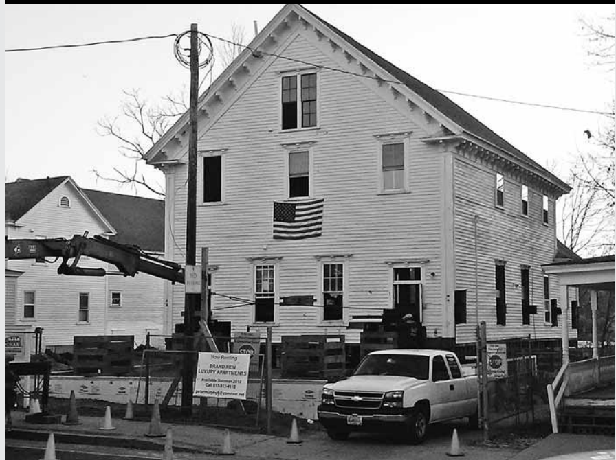
In early November, the historic Grange structure was moved forward to a new foundation adjacent to the sidewalk on Main Street. Photo Courtesy of Todd I. Selig
