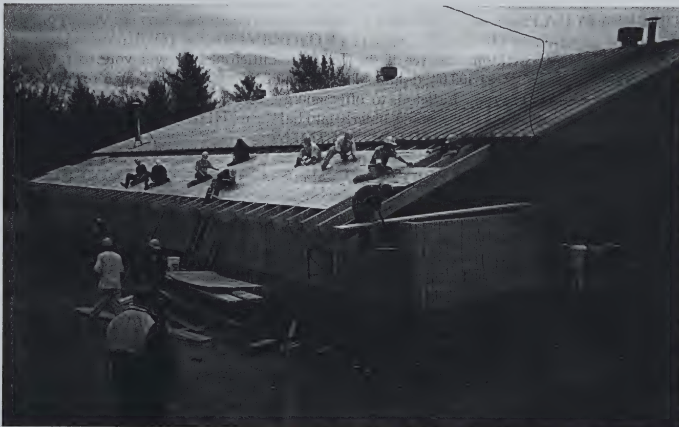
Students from the Hugh J. Gallen Vocational Center work on the addition to the Town Garage in the fall of 1999. This was a result of the passage of Article 6 at Town Meeting
