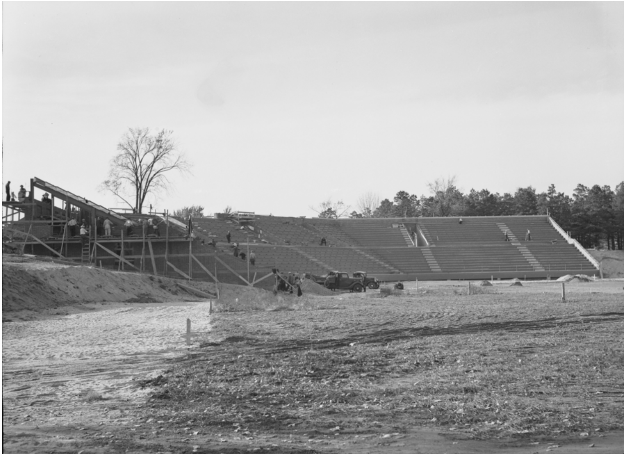
Municipal Stadium (Holman Stadium) Being Built by WPA – 1936 National Archives – Negative 5295-A, New Hampshire, Athletic Fields
