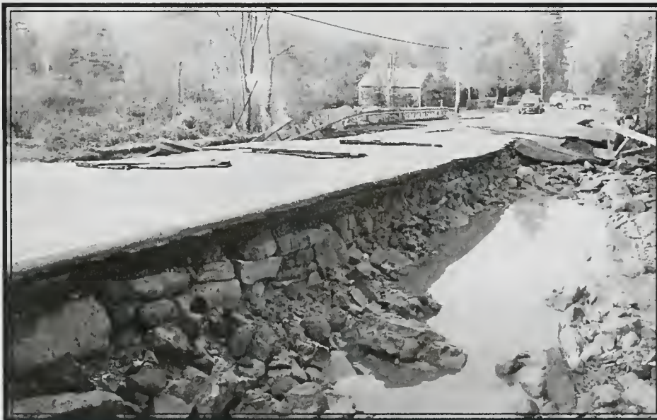
Hamel Brook located south of Laurel Lane on Route 108 after the flooding on May 13 and 14, 2006. PHOTO COURTESY DEPT OF PUBLIC WORKS
