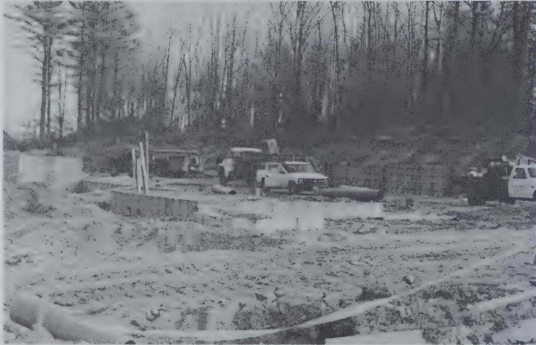
Capitol Plumbing and Heating begins construction of a sq. ft. structure in Enterprise Park.
