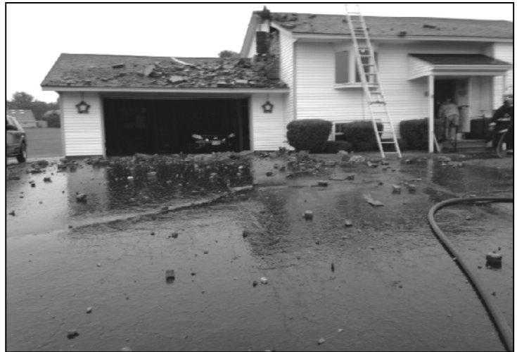
Lightning Damage – Countryside Drive
