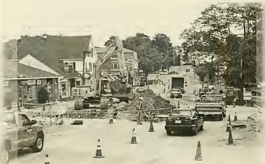
Two views showing Main Street under construction for the Downtown Main Street Enhancement Project.
