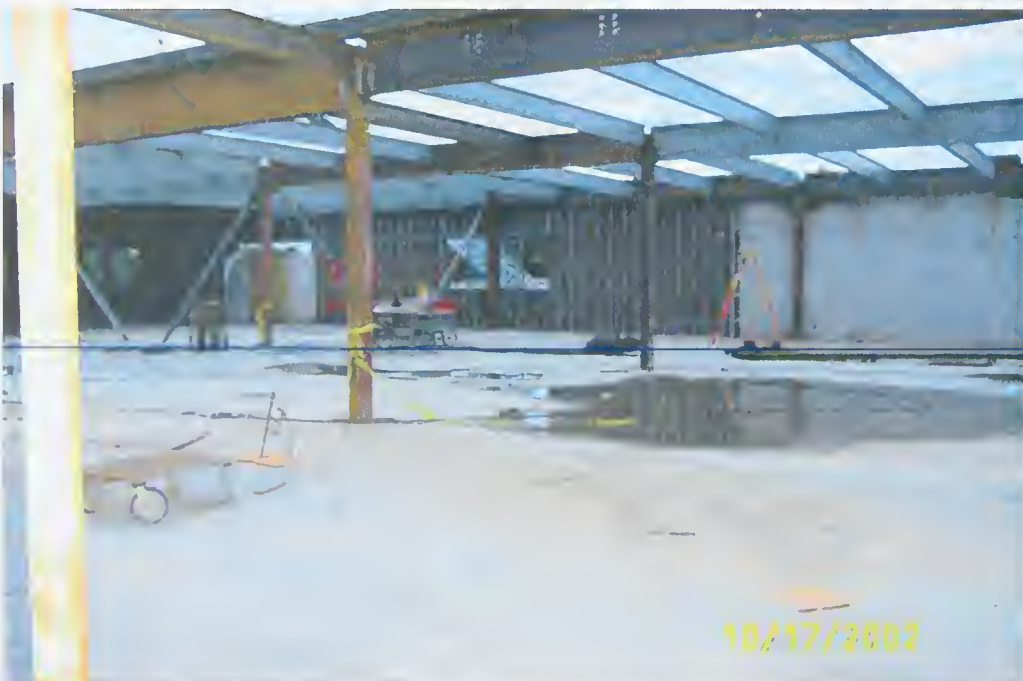
This photo shows the work underway in the former "A" wing, which is being renovated into classrooms and academy offices. photo by Richard D. Burpee
