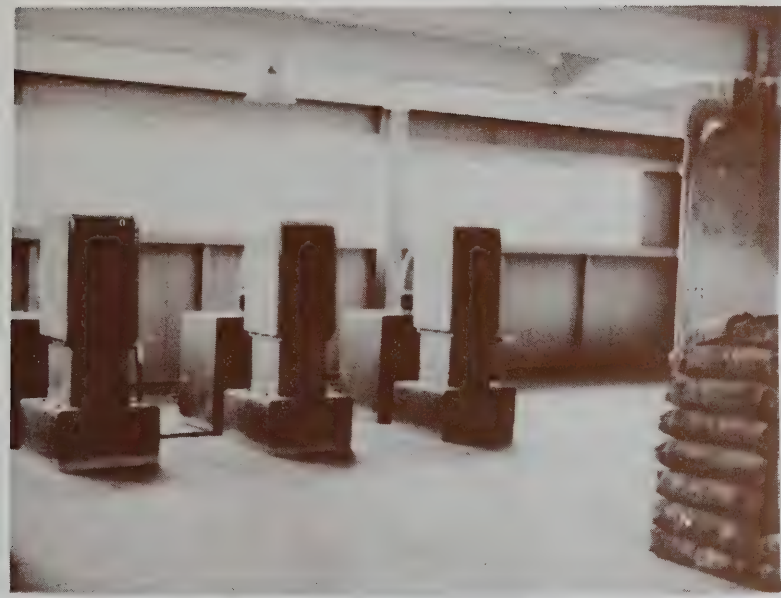
Feeders — Chlorine, lime and alum — used in treating surface water to State Water Pollution Commission requirement.
