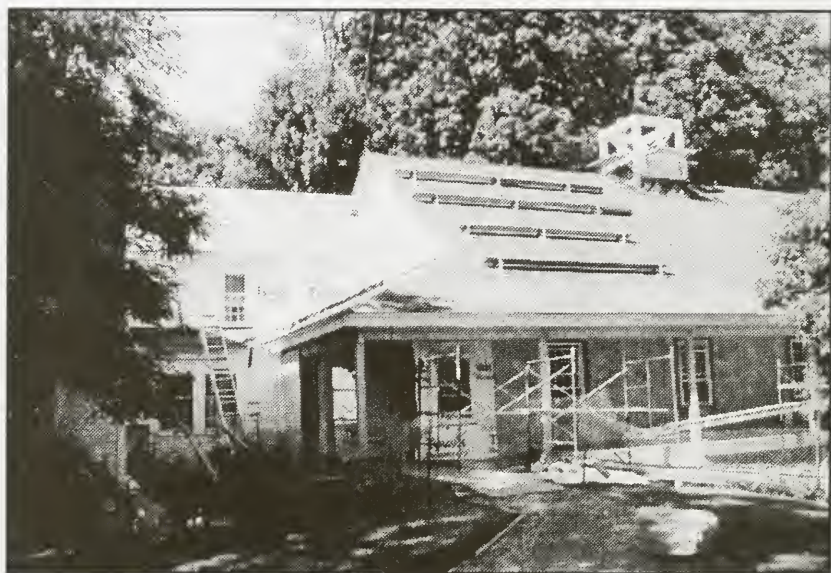
The porch is up and the roofing almost complete. Work on the cupola has started.
