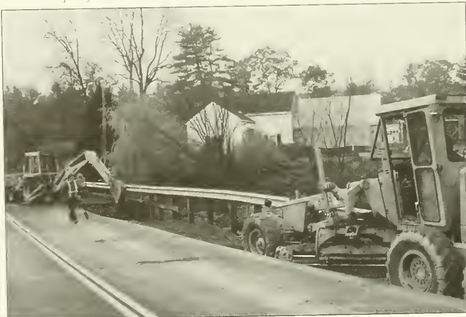
Repair of Rt. 108 at Hamel Brook, October 1996. (photo courtesy Michael D. Golding)
