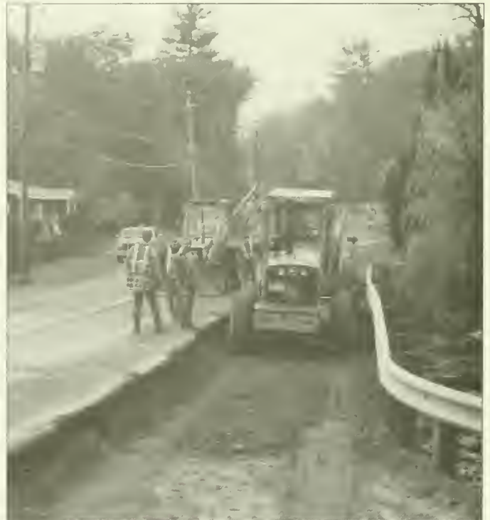
State crew workers repair Newmarket Road washout at Hamel Brook, October 1996. (photo courtesy Michael D. Golding)
