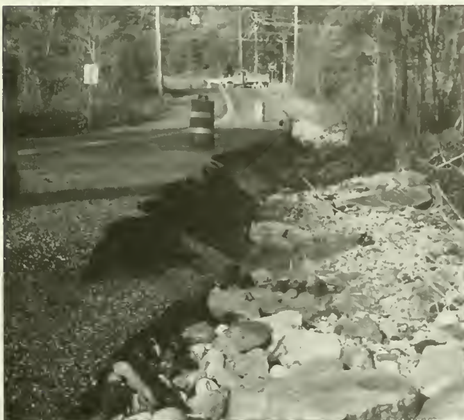
A portion of Longmarsh Road damaged by the flood, October 1996. (photo courtesy Richard H. Lord)
