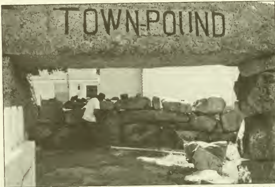
The Town Pound, nearing completion after skillful masonry work of John Wastrom (pictured) and assisting masons William and David Allen (not pictured).
