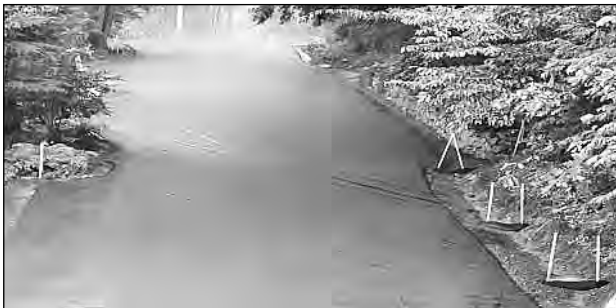
Photograph of the end of Lake Avenue in Georges Mills. This section of road was ground, regraded such that stormwater flowed away from abutting properties and Lake Sunapee, and into new paved swales and a cast-in-place catch basin at the low point of the road for improved stormwater treatment.
