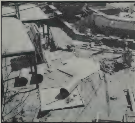
No longer a parking lot, Bicentennial Square plaza slowly assumes shape. (Concord Monitor photo)
