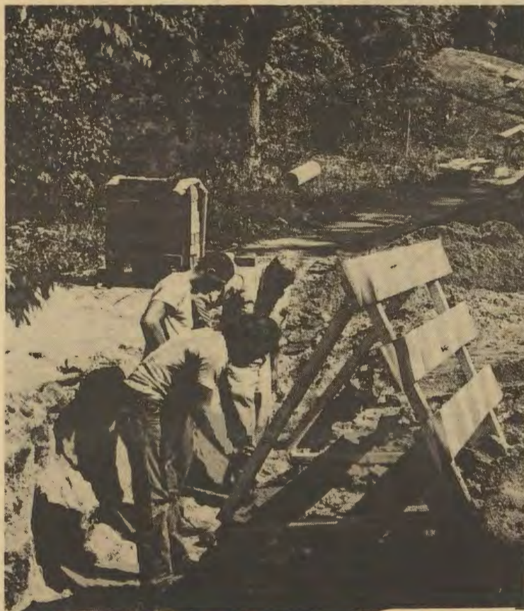
Work will continue for about five more weeks on Garrison Ave. as sidewalks, ramps and bike paths are constructed. (Steven Morrison photo)
