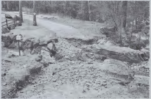
The damage left after Whittemore Lake exceeded the dam's capacity. The spillage washed away Whittemore Lake Road West
