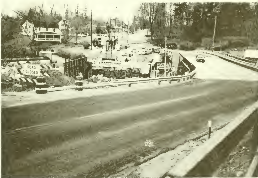
A rare sight during construction — just one car crossing the bridge during business hours!
