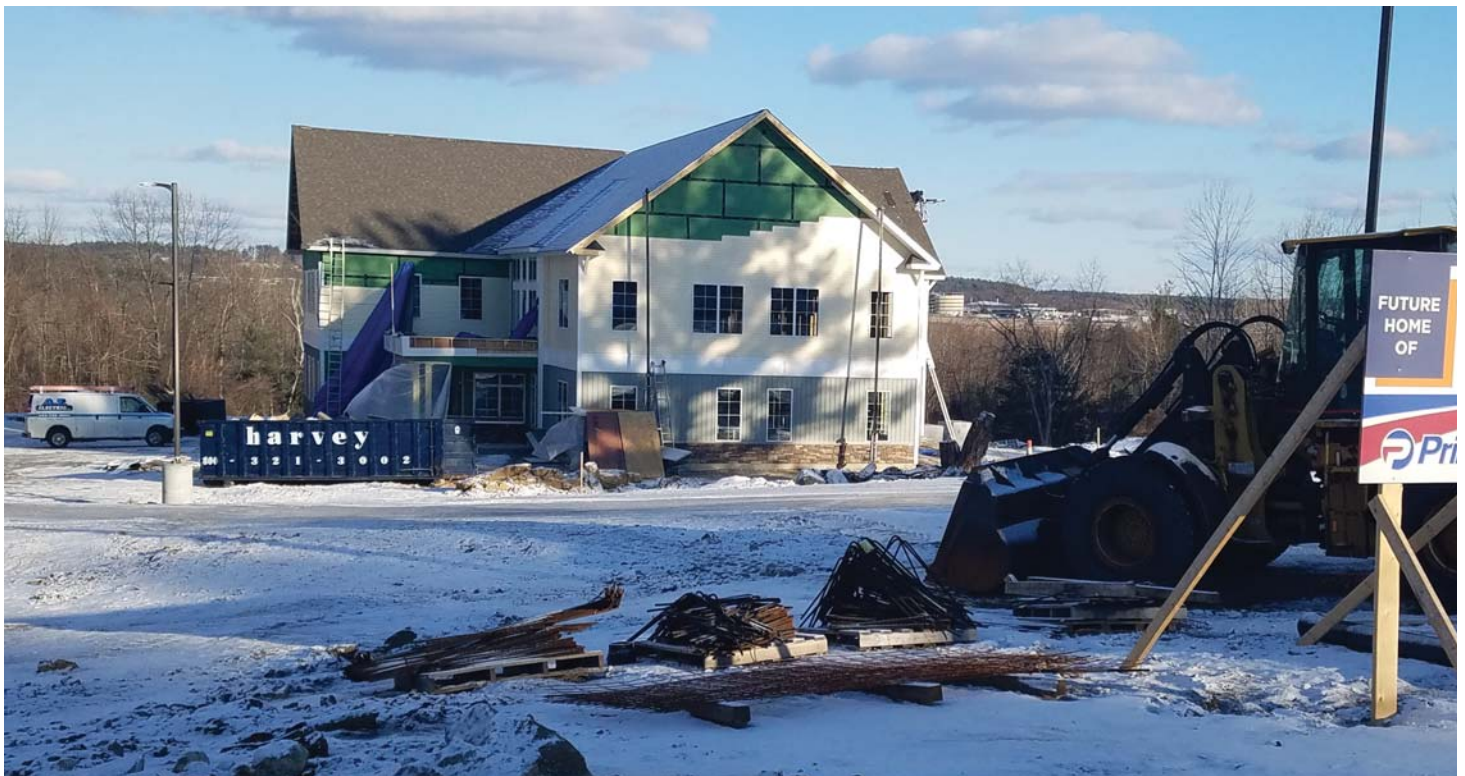
A new office building for The Harbor Group Inc., a financial planning company, was one of several development projects under construction along South River Road in late 2017
