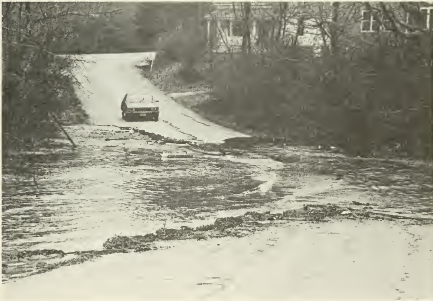
Damage from 1987 Flood on Bennett Road.
