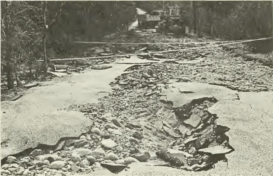
Damage from 1987 flood on Bennett Road.
