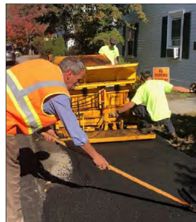
Highway Team members Perkins, Batchelder & McCallum use the sidewalk paver on Elm Street.
