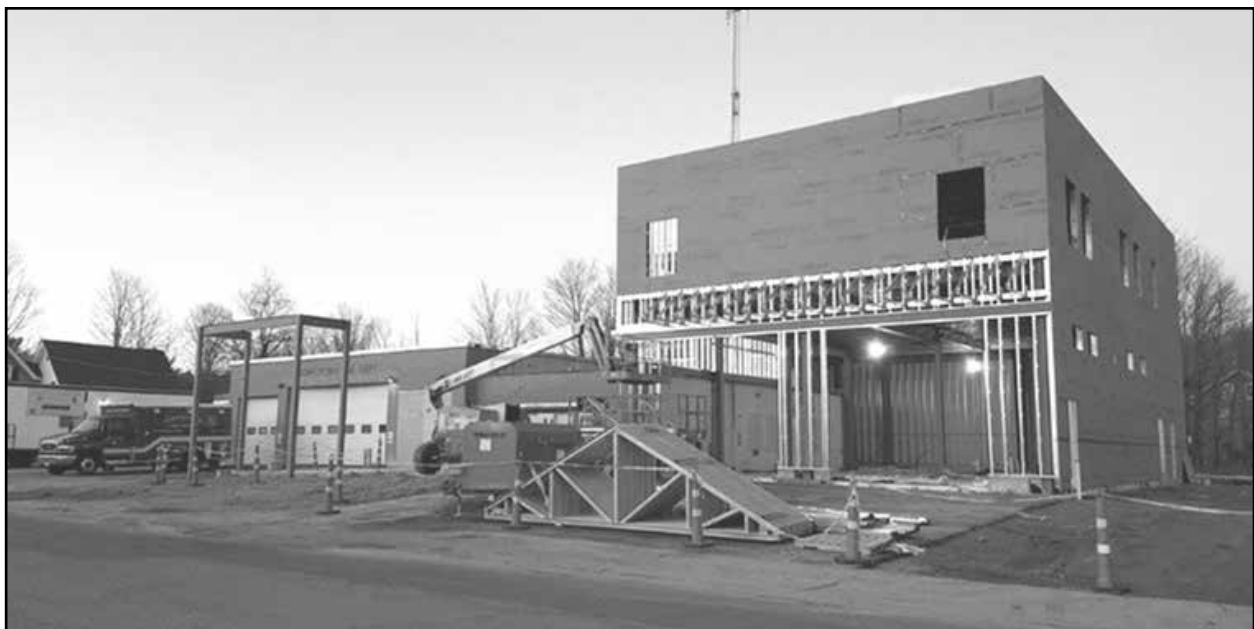
After the ground breaking ceremony, construction of the fire station quickly commenced. Note: The fire station stayed operational during construction.
