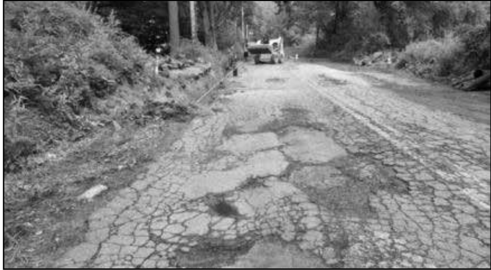
The pavement was well beyond its useful life on Worthley Hill Road.
