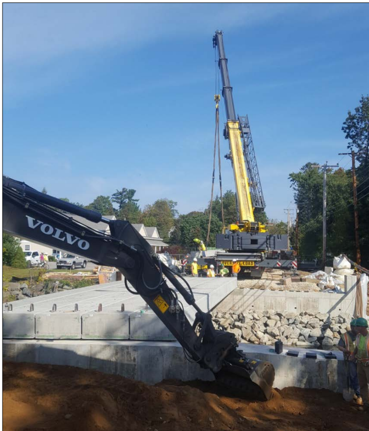
Court Street Bridge construction at Little River. Photo by Jay Perkins, Sr.
