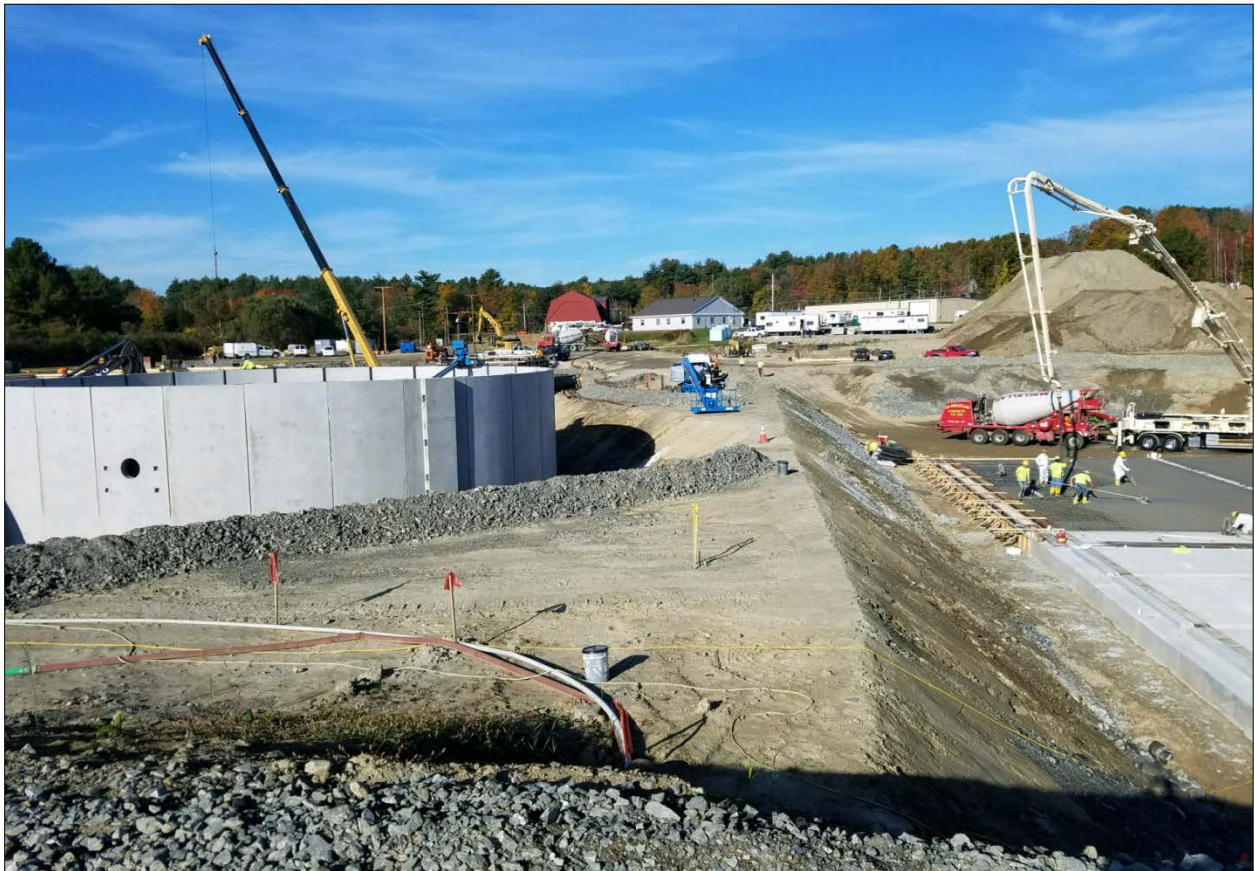
Wastewater Treatment Facility construction at the Newfields Road site. Photo by Matthew Berube
