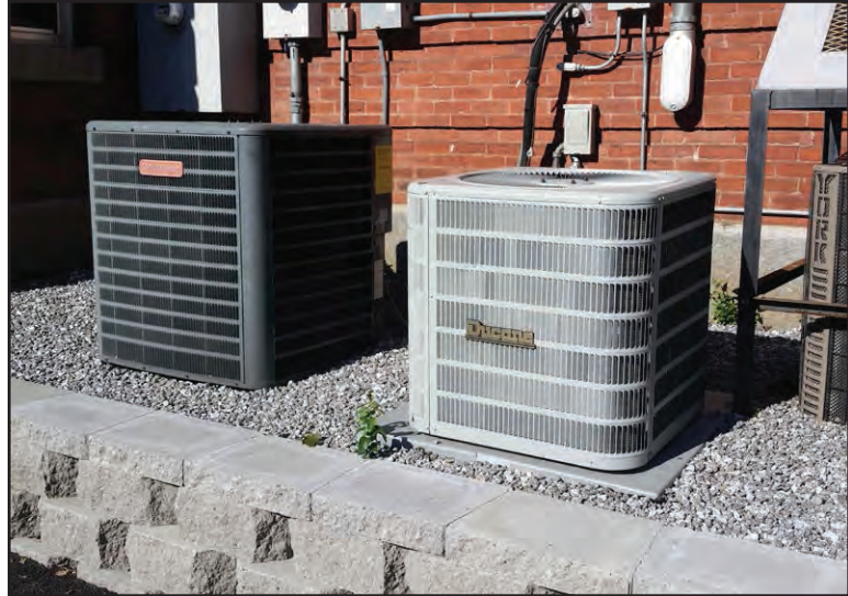
Children's Room - Central Air Conditioning Project Condenser Unit & Retaining Wall
