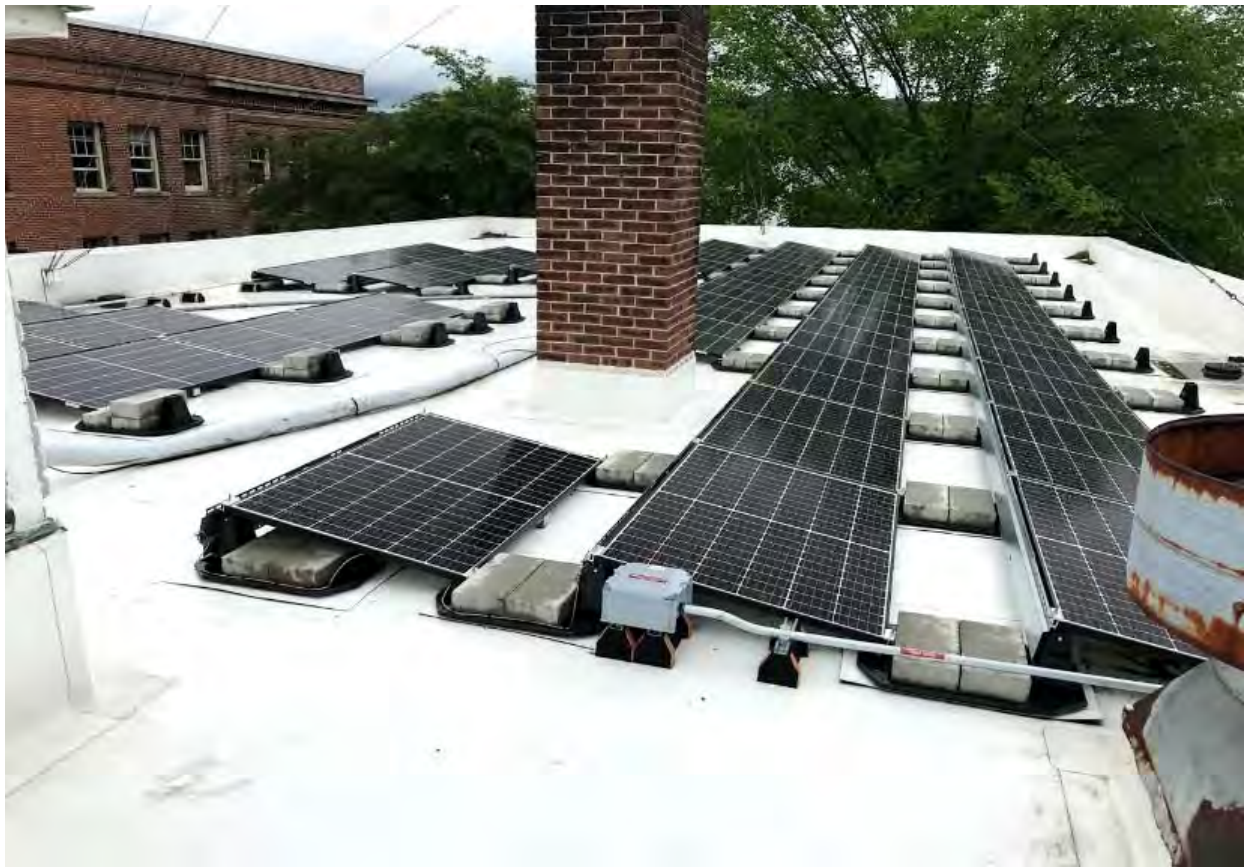
Solar Array at Town Hall
