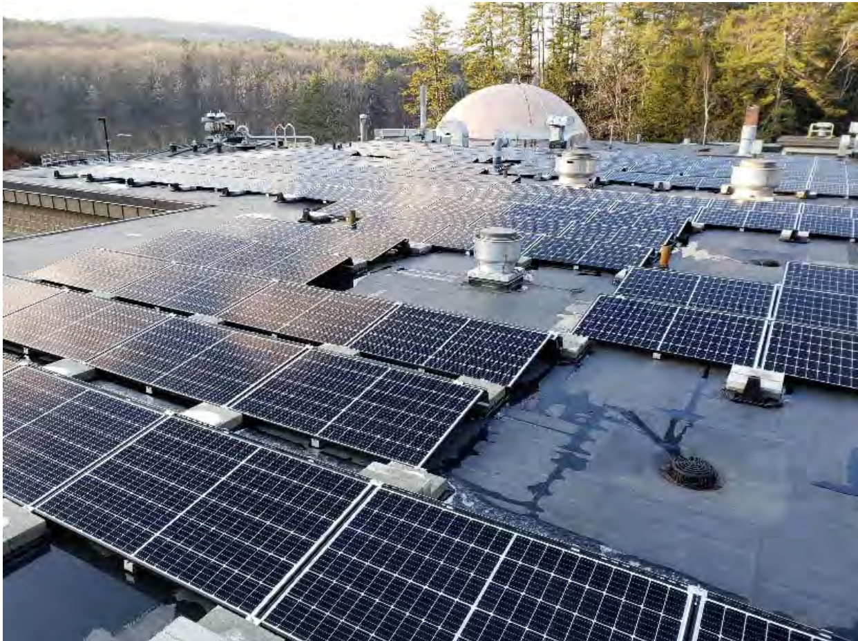
Solar Array at the Water Reclamation Facility
