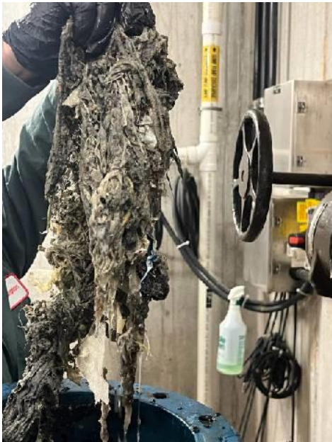
“Wipes” clogging the Church Street Pump Station
