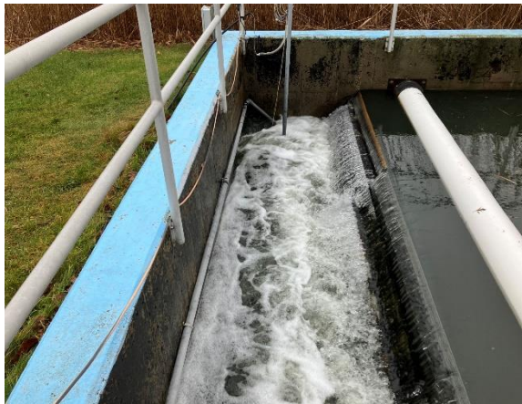
WWTP Chlorine Contact Chamber
