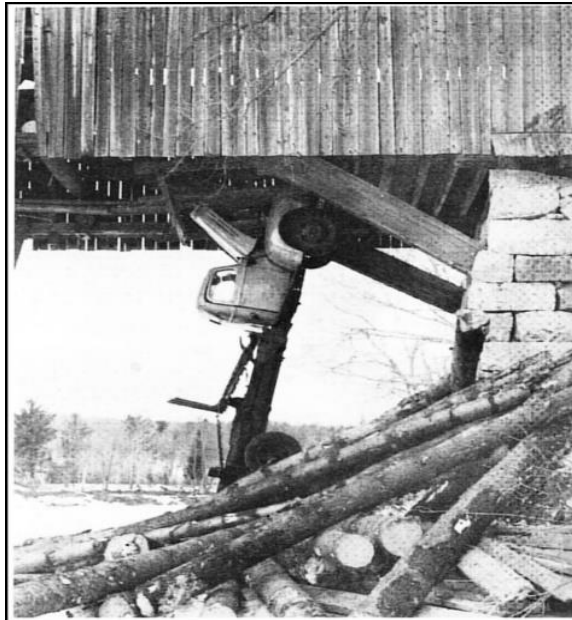
Logging truck that fell through the Blair Covered Bridge
