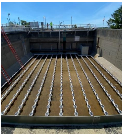
New Aeration Basin Diffusers
