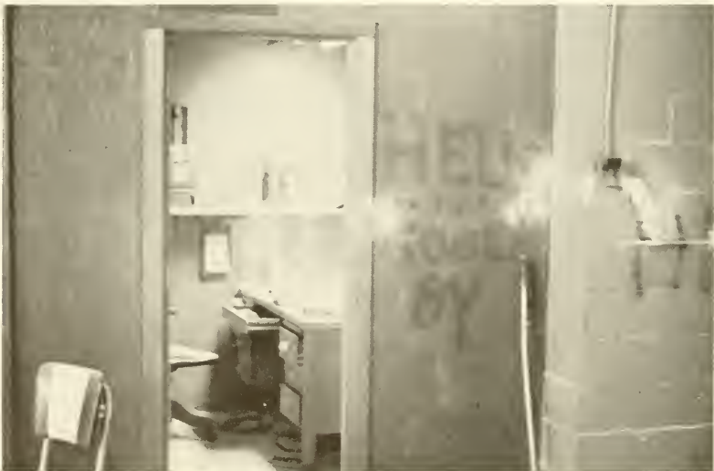
Vandalism at Incinerator
