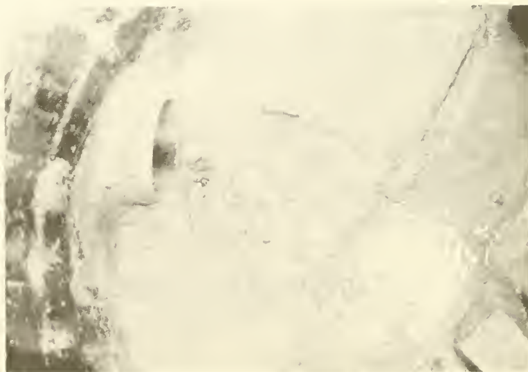
Poorly Constructed Manhole
