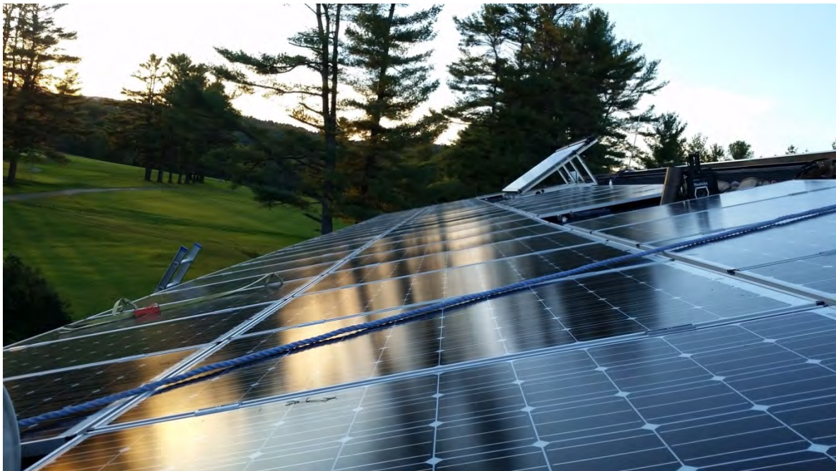
Solar Array on Police Department Roof
