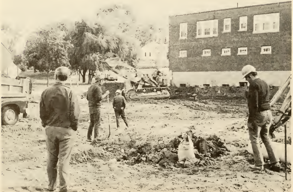
This is what the Parking Lot looked like after clay was removed.....
