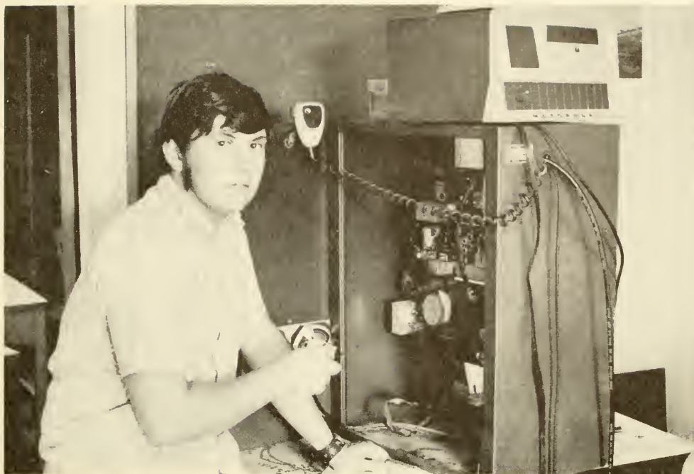
Student Peter George installing surplus Police radio system in the Highway Department
