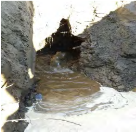
Leaking service line
