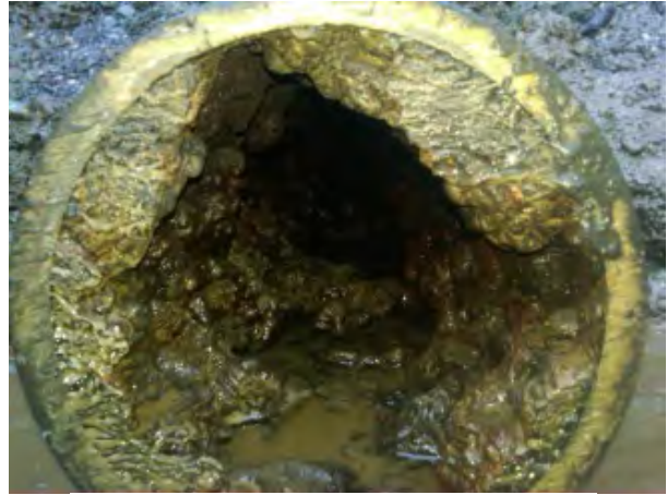
Old tuberculated water main
