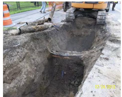
Direct bury electrical cable
